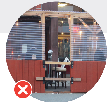
This is a non-compliant gap because of the overhead and pathway obstructions.
