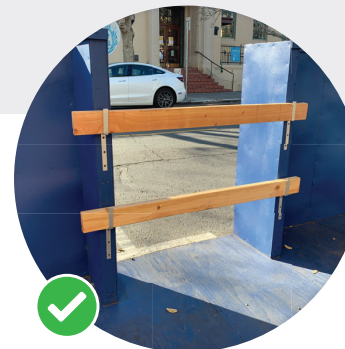
Provide a rigid, easily-removable barrier at the 3-foot gaps.
