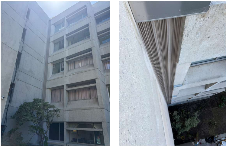
West Façade 25" Vertical Seismic Expansion Cover
