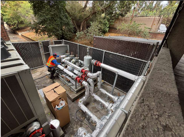
Insulated chilled water lines
