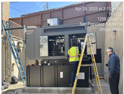
New Generator at FS 44
