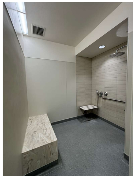
Completed Commuter Shower
