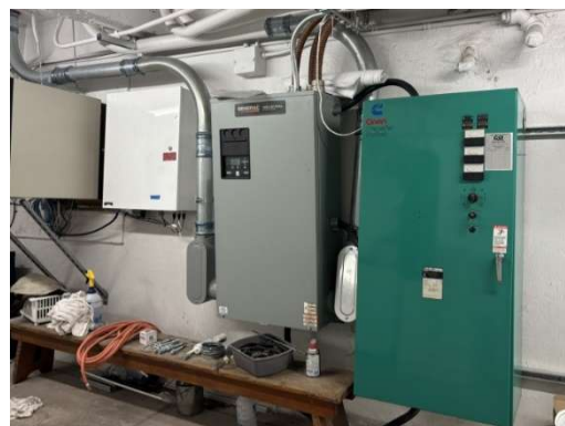
New Generator Electrical Panels at FS 44
