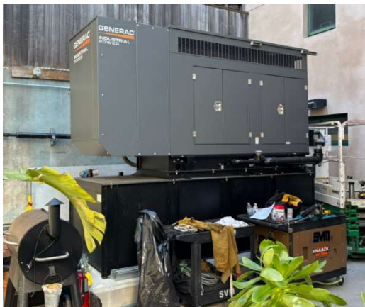
New Generator at FS 37
