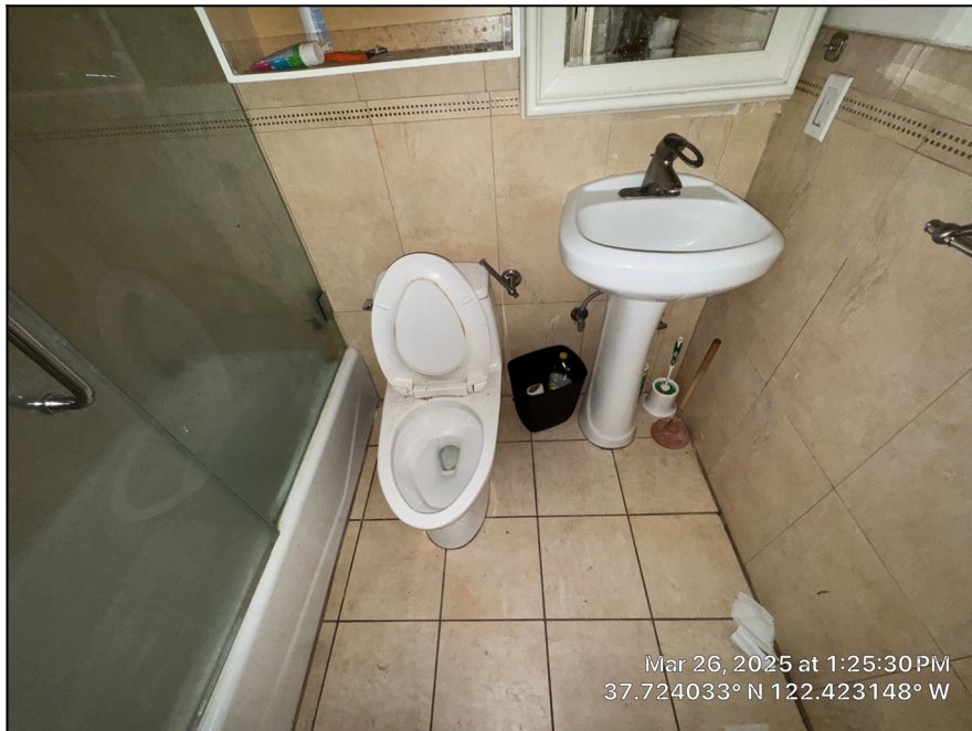
Figure 12. Second-floor bathroom receptacle located within two feet of the pedestal sink.
