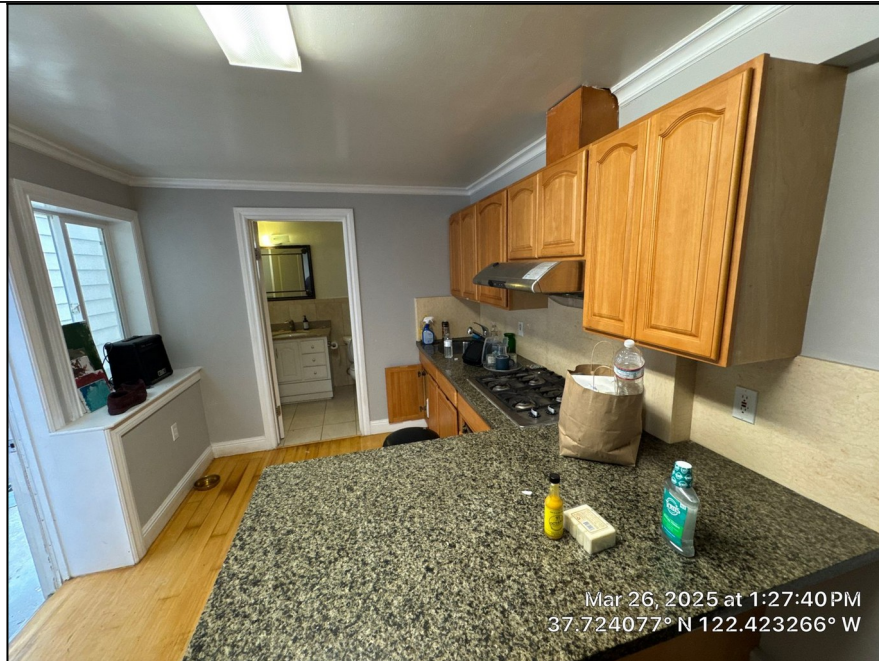
Figure 3. Unpermitted kitchen on the ground floor, with cabinetry, gas cooktop, and a bathroom beyond. The ground floor is approved only as family room, bathroom, and storage (S.F. Housing Code §301).
