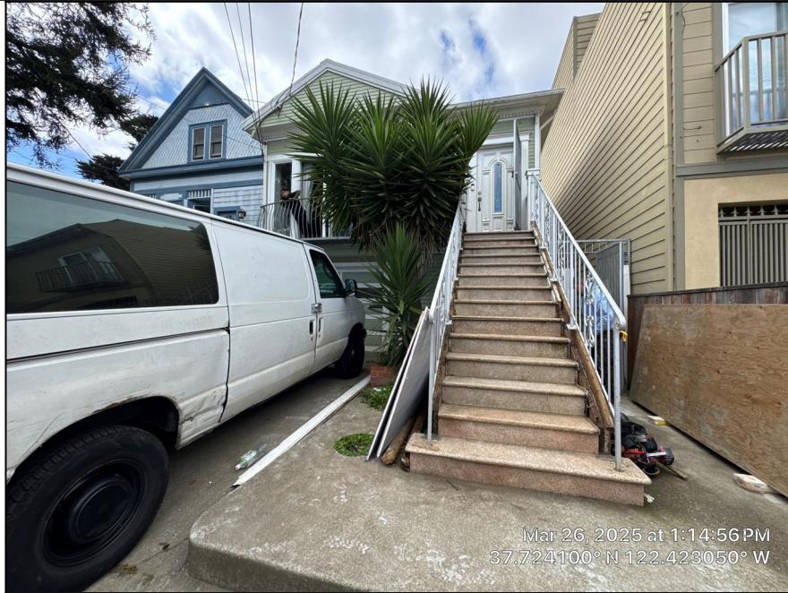
Figure 9. Front entry stairway, the building's only means of access, with deteriorated wood at the top landing.
