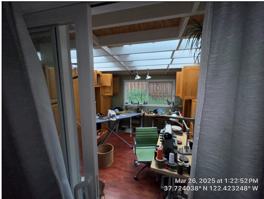
Figure 6. The enclosed rear room created from a former porch, covered by a translucent plastic roof. It has no exit to the exterior and no proper light or ventilation (S.F. Housing Code §504).
