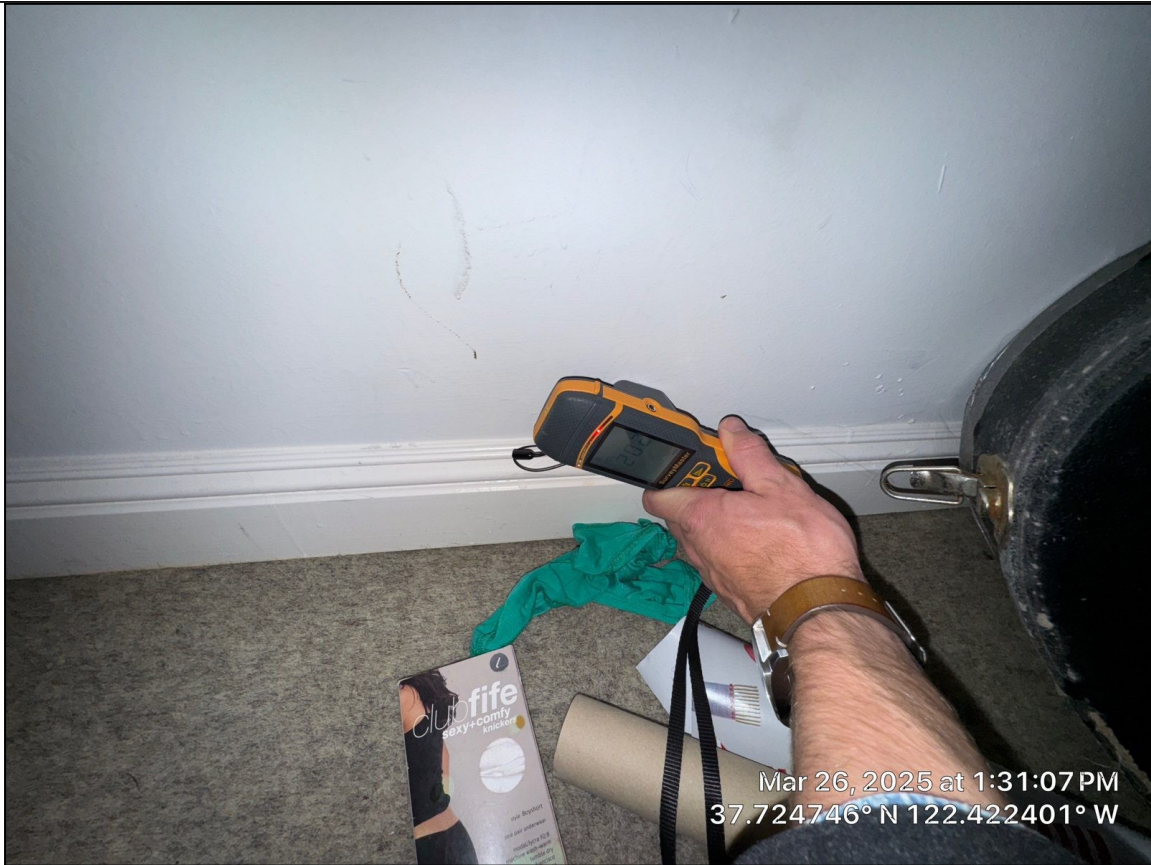
Figure 15. Moisture meter against the lower edge of a wall in the rear storage area, recording elevated moisture consistent with water intrusion (Cal. H&S Code §17920.3(a)(11)).
