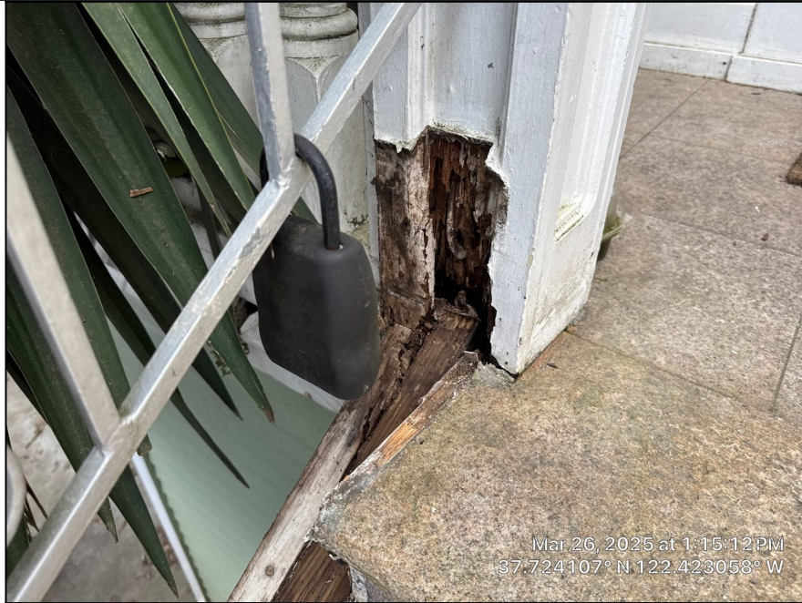
Figure 11. Close-up of the left side of the entry landing, showing wood rotted through to bare, splintered material (Cal. Civ. Code §1941.1(a)(8)).
