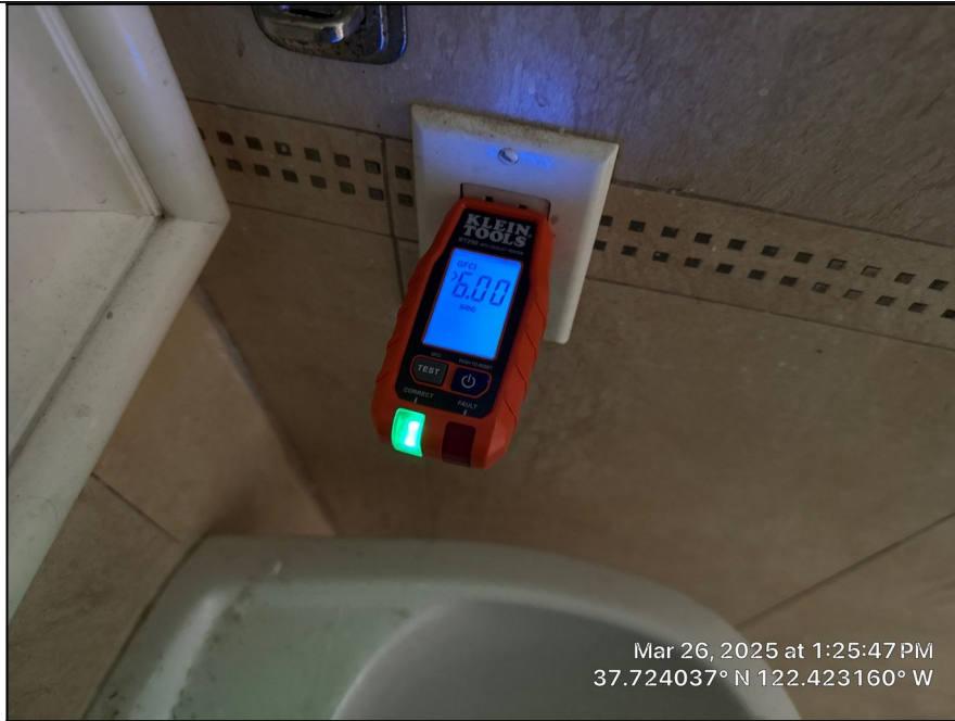
Figure 13. Klein Tools GFCI tester at the same receptacle. The tester ran a full six seconds without tripping, confirming no ground-fault protection (Cal. Elec. Code §210.8(A)).
