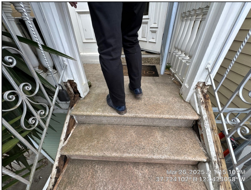
Figure 10. Top landing of the entry stairway. The wood framing on both sides is severely dry rotted and deteriorated.
