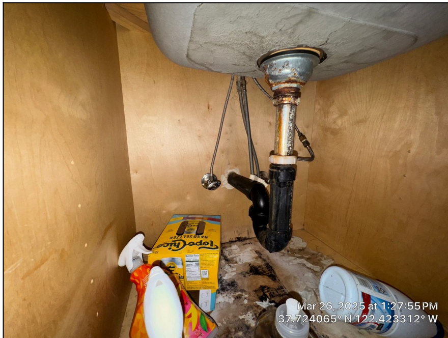
Figure 14. Plumbing beneath the ground-floor unit sink: a corroded drain and active leak with staining and water damage to the cabinet base (S.F. Housing Code §1001(f)).
