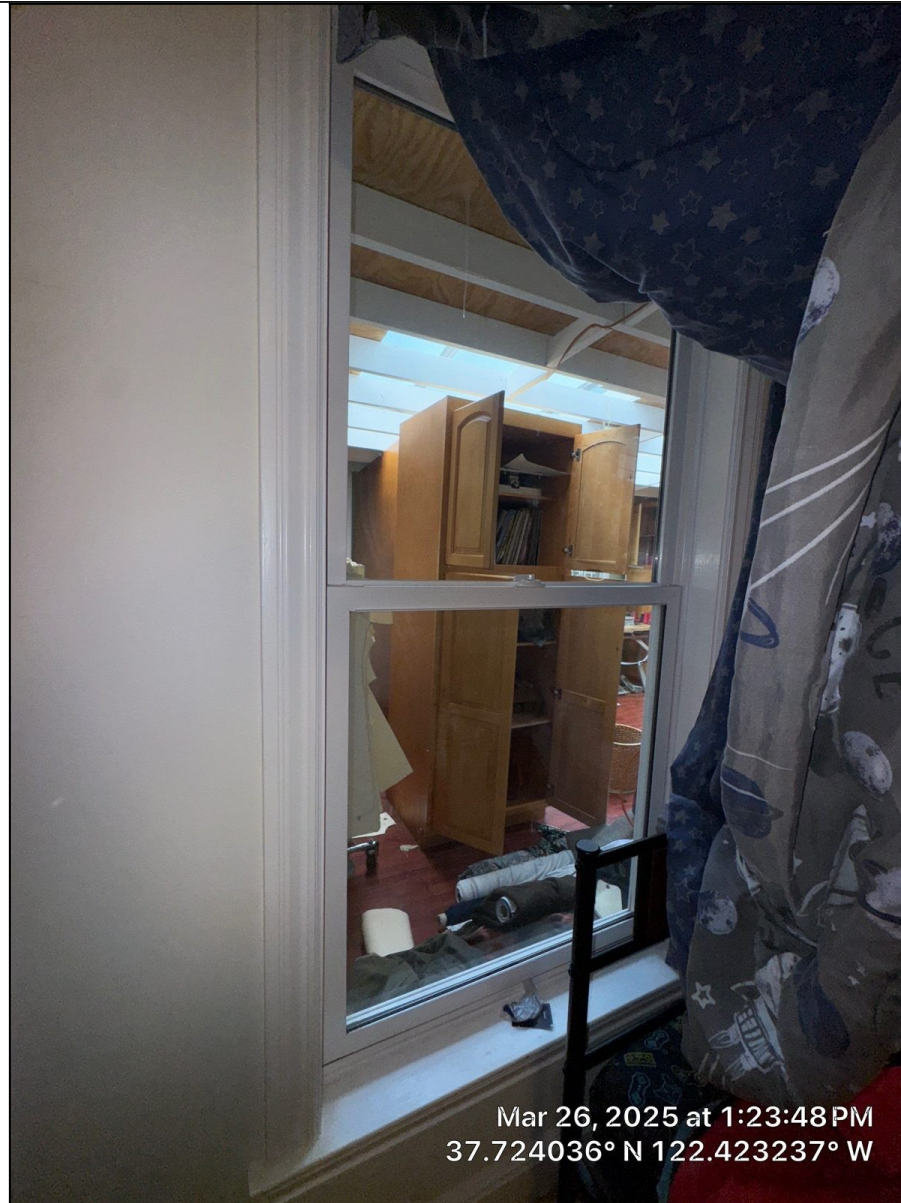
Figure 8. Window of the rear left bedroom opening into the enclosed deck rather than to open air, providing no emergency escape, light, or ventilation (Cal. H&S Code §17920.3(l)).
