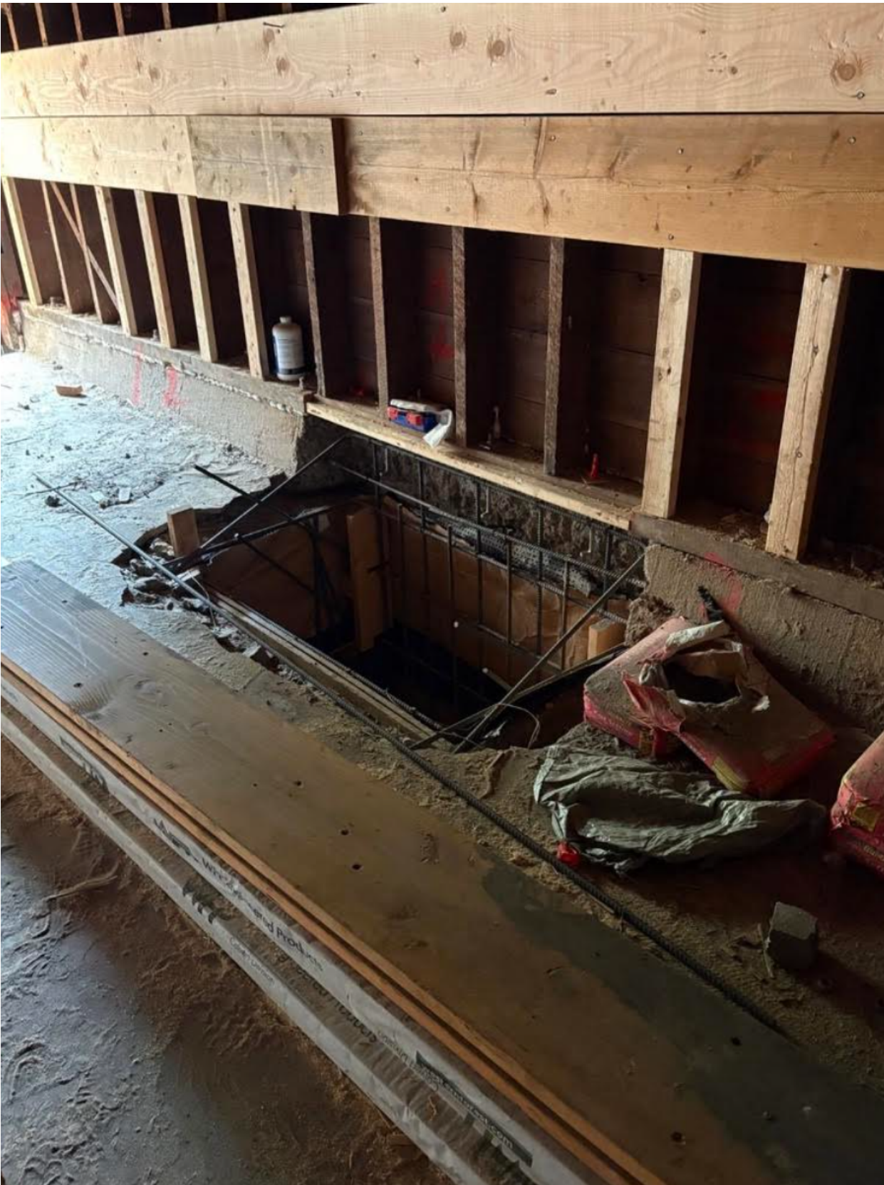
EXHIBIT 03 Image shows the same excavation pit located in the middle of the house.
