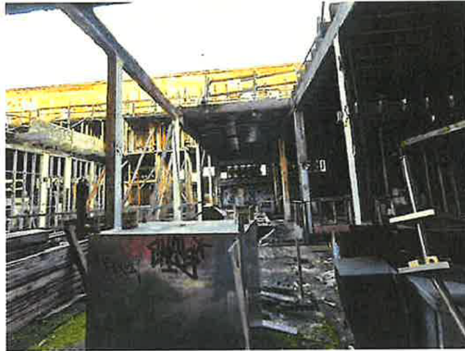
Missing Roof and Floor Diaphragms 02/04/2025
