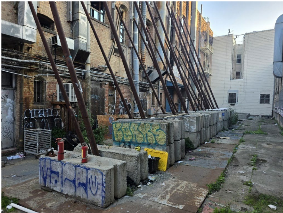
Rear Yard Out-of-Plane Wall Bracing System
