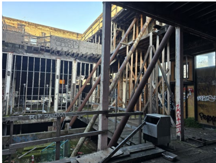
Missing Roof and Floor Diaphragms 02/04/2025
