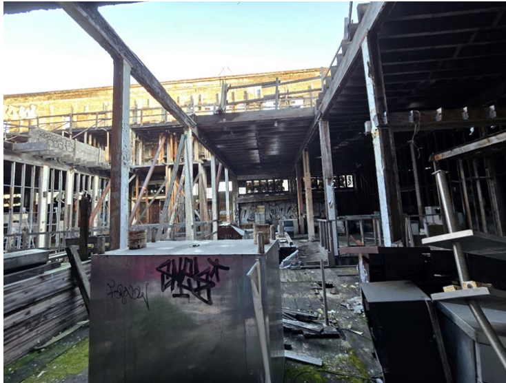
Missing Roof and Floor Diaphragms 02/04/2025
