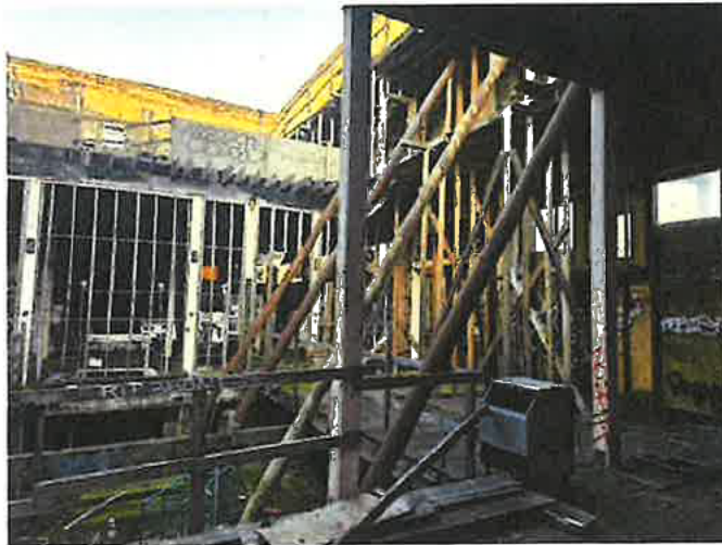
Missing Roof and Floor Diaphragms 02/04/2025
