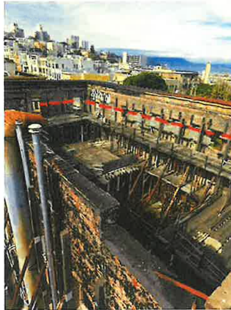
Likely location of flexural failure
