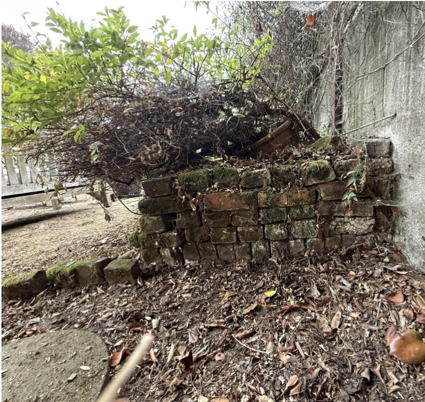
Green growth on bricks used to continue to wall. Growth on wall and closest bricks has died off, along with plants.
