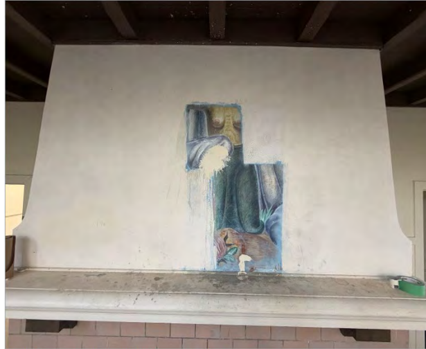
Figure 66: Overall view of the first-floor fresco before treatment.
